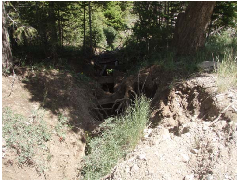
Photo#31 Caved adit of the Allie Tunnel along side of the public road. (B. Schuld 7/22/10).
