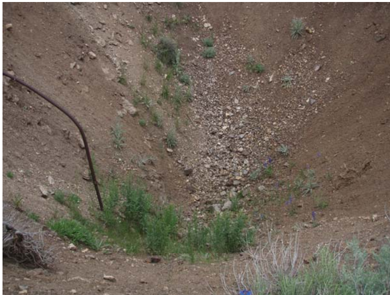
Photo #7 Collapsed Shaft on Latest Out Waste Dump (B. Schuld 7/22/10)
