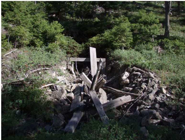
Photo#37 Dangerous opening of the Dorothy Tunnel adit. (B. Schuld 7/22/10).
