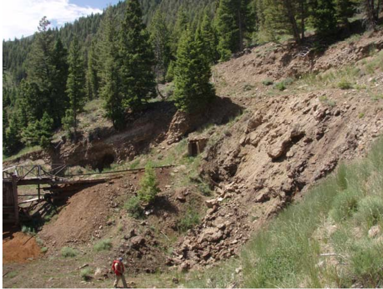
Photo #21 Three dangerous open adits remain on the Silver Dollar. There as apparently some redevelopment work that was conducted on these adits and a small ore bin/chute was constructed to ship some ore or bulk samples (B. Schuld 7/22/10).
