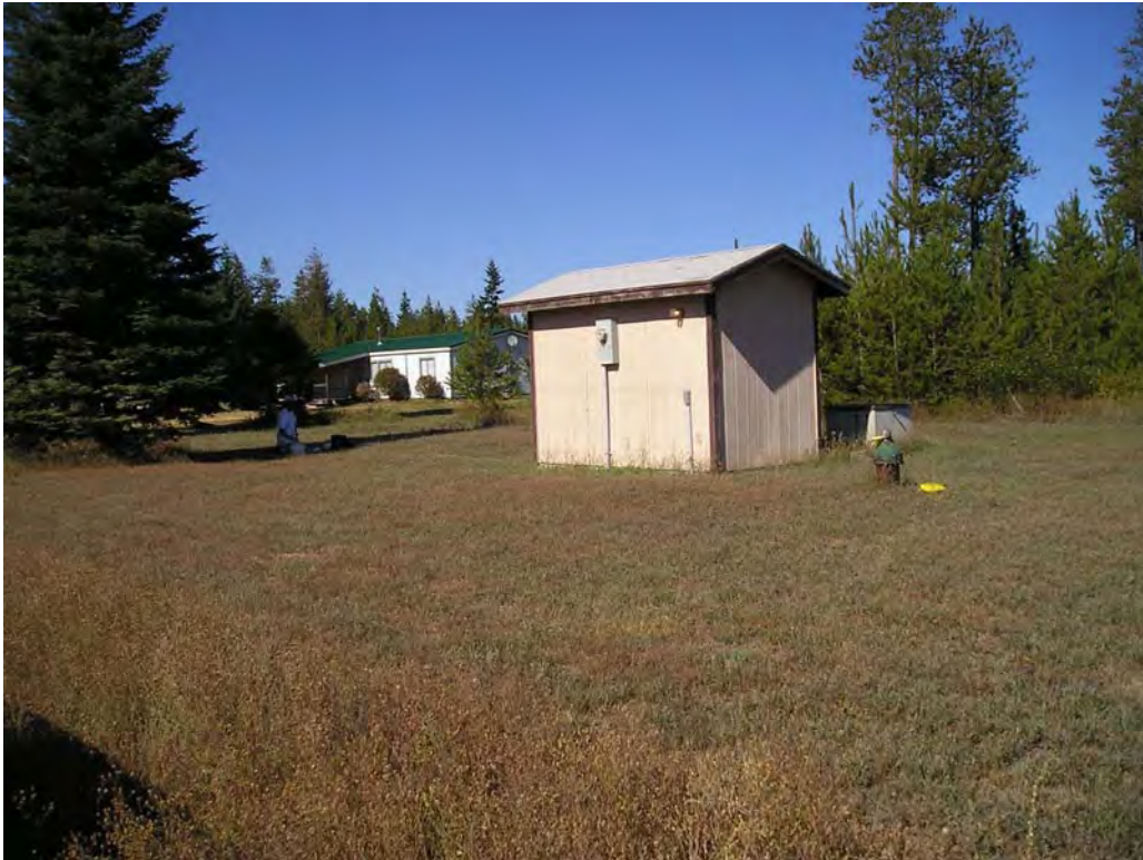
Figure 5. Photo showing a typical community water supply well head and building housing pressure tanks and distribution equipment.
