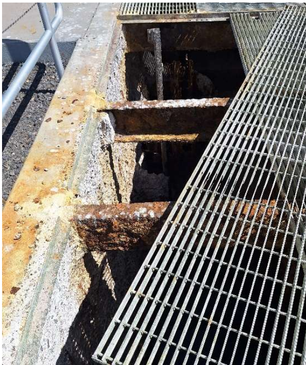
Figure 3. H 2 S corrosion in WWTP influent channel.
