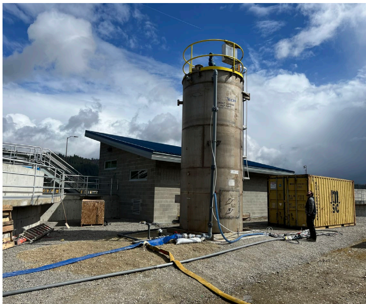
Solids contact clarifier pilot unit and control building
