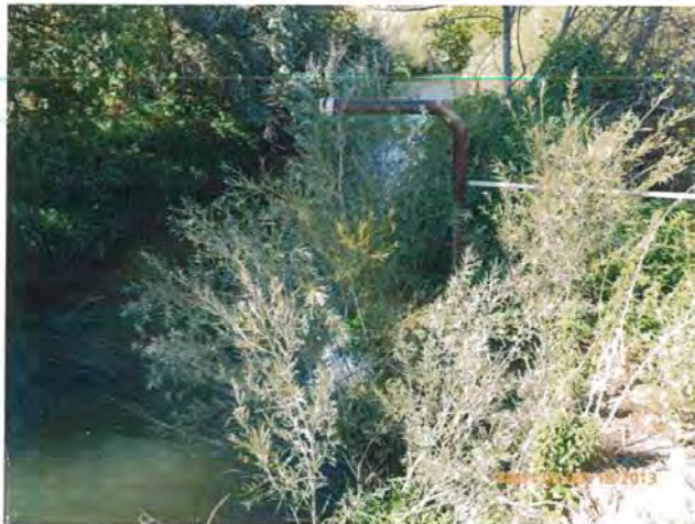
Photo No. 7 (P1000206) The non-contact cooling water flowing from the water cooled condenser is discharged to Rock Creek at this location.
