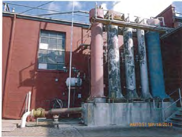
Photo No. 6 (P1000203) Cooling water enters the top of the five-tower water cooled condenser and flows from the cement tank at the bottom.
