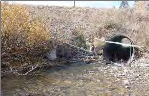
Targhee Creek Culvert under Highway 20 before replacement was a barrier to upstream-migrating Yellowstone cutthroat trout.
